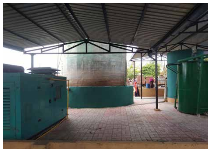
Bio-Methanation Plant at Madri Station, Udaipur
