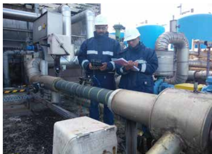
Energy audit at Indorama Europort, Rotterdam, Netherlands
