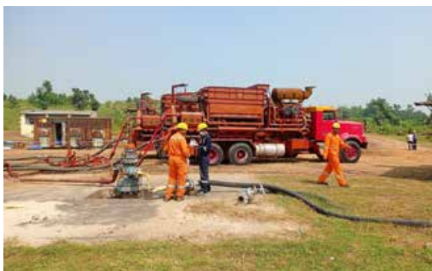
▶ Application of coal bed methane (CBM) technology in CBM wells
