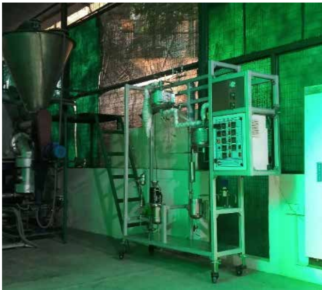
▶ Bio oil catalytic upgradation unit
