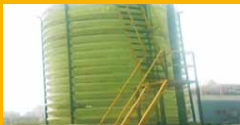
Natural Cooling Tower
