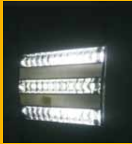
Before with 3X36Watts CFL light fixture
