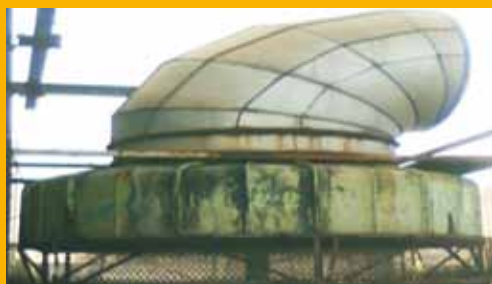
Forced Draft Cooling Tower
