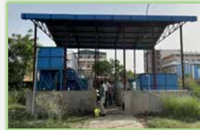
ONSITE PLANT: 20 KLD TADOX® Plant in 100 sq ft space, in Textile CETP in Kanpur funded by NMCG, MoJS, GoI
